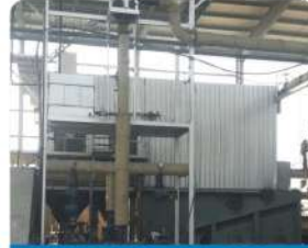
BIOMASS THERMAL OIL HEATING SYSTEM
