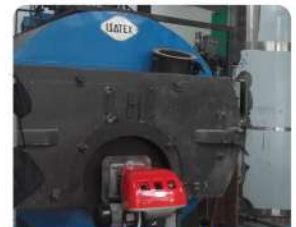
DIESEL FIRED STEAM BOILER
