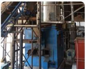
BAGASSE FIRED HIGH PRESSURE THERMOSYPHON
