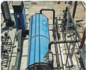
FUEL OIL FIRED THERMAL OIL HEATER
