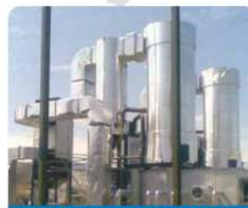
BIOMASS FIRED THERMAL OIL HEATER SYSTEM
