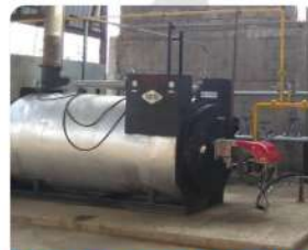
FUEL OIL FIRED THERMAL OIL HEATING SYSTEM
