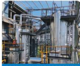
COAL FIRED HIGH PRESSURE THERMOSYPHON
