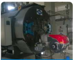
GAS FIRED STEAM BOILER
