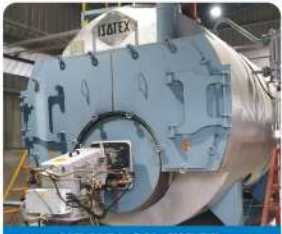
HEAVY OIL FIRED STEAM BOILER
