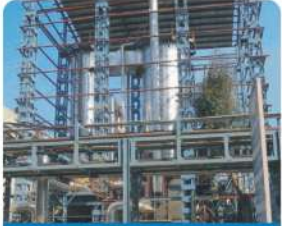
COAL FIRED FBC THERMAL OIL HEATING SYSTEM
