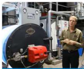
FUEL OIL FIRED THERMAL OIL HEATING SYSTEM
